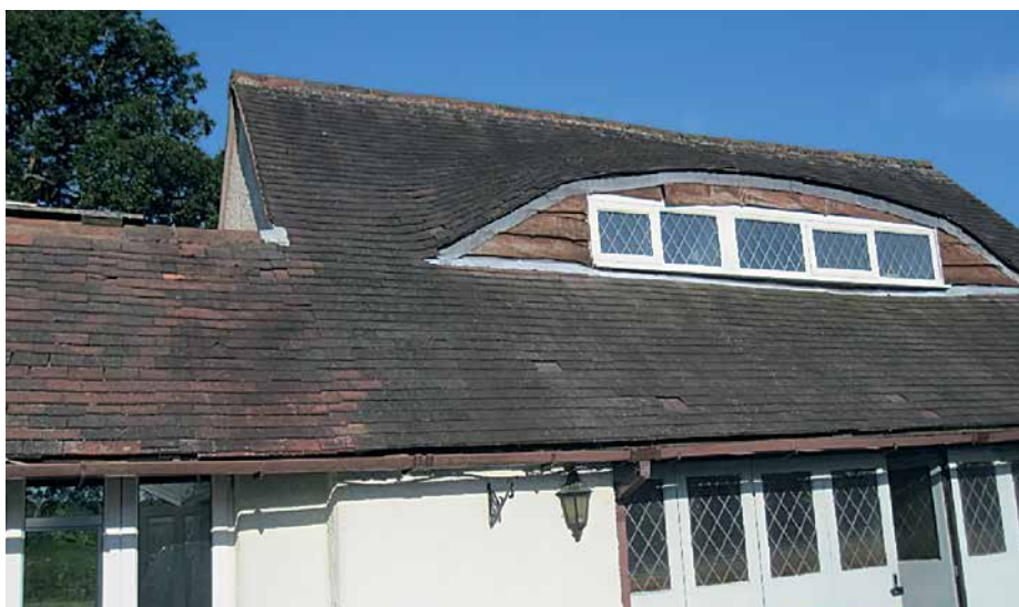
This house, located in an area of excellent bat foraging habitat, with slipped/missing roof tiles and gaps beneath weatherboarding/lead flashing leading to voids behind, was deemed to have "negligible bat potential" by a surveyor. Photo credit Lisa Kerslake.
